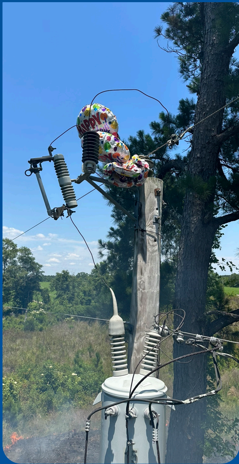
Excelsior EMC Serviceman, Jody Wilson, took this picture of a helium balloon that got caught in a power line and caused an outage, as well as the ground fire that can be seen in the bottom left.
