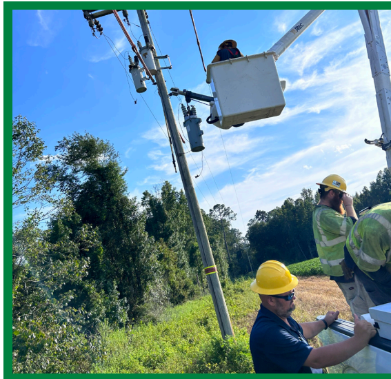
Retired Excelsior EMC employee, Jessie Goodman, and a Pike Electric crew work to replace a recloser on a three phase line.
