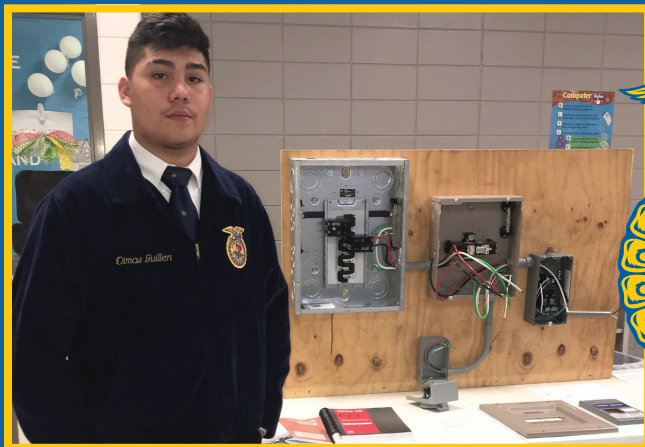
Dimas Guillen explains the operating principles and installation for a manually operated transfer switch used in conjunction with a generator on a storage building.
