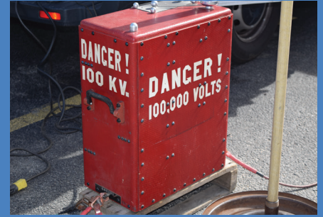
This testing transformer produces up to 100,000 volts of electricity!
